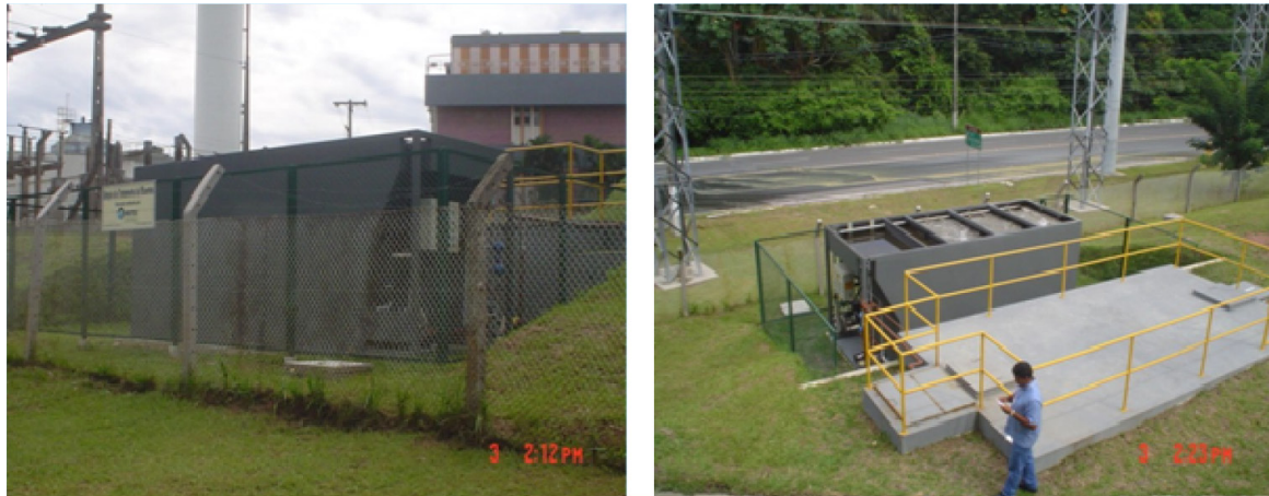
Figure 1. Examples of fixed EEC High-Speed Bio Tec – 120 m 3 /day treatment plants.
