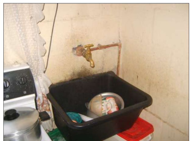
Figure 7. An example of a kitchen area in Greenfields. Note the rudimentary facilities and dirty wall. This is the only working tap in the main house.
