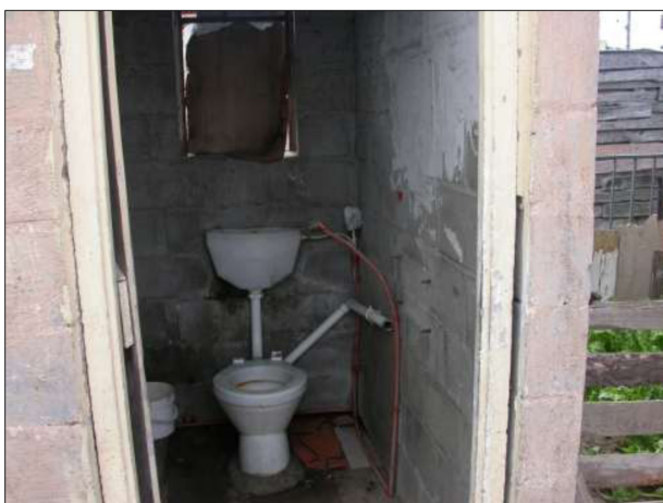
Figure 5. Tap against the wall on right is either lost or removed. Note the broken pipe and cistern, as well as the broken window which has been repaired with cardboard in Masipumelela.
