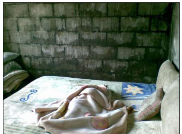
Figure 3. Dampness penetrating bedroom wall with infant sleeping on bed in a low-cost house in Greenfields.
