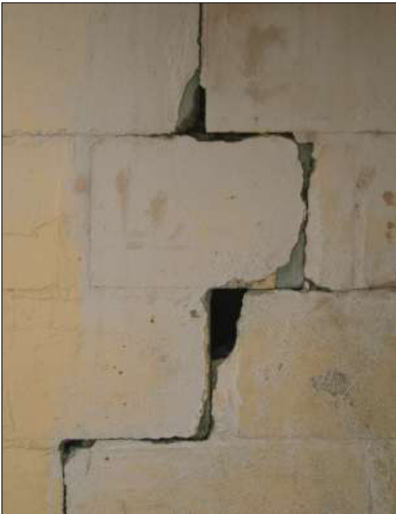
Figure 4. An example of structural damage: a seriously cracked wall of main house in Tafelsig.
